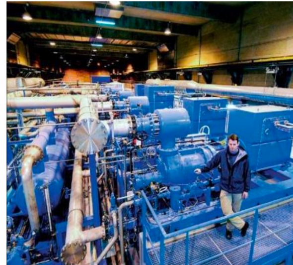
One of the 8 compressor units of the 4.5 K refrigerator for LHC
